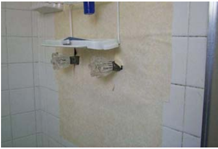
Figure 4. Improper tile and grouting repair.
