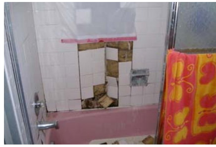
Figure 5. Total collapse of the shower wall.
